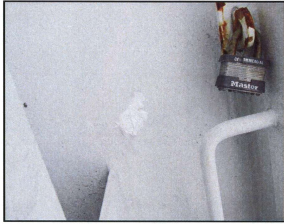
Roof access hatch locked
