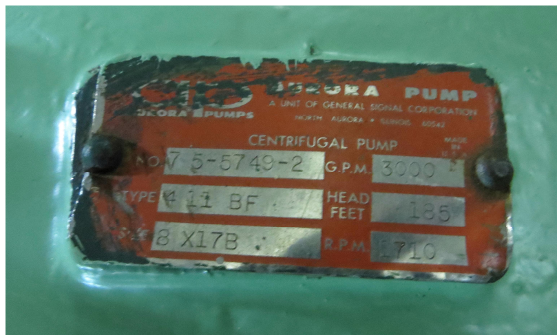
RESTON PUMP STATION'S PUMP #1 NAMEPLATE
