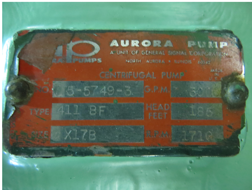
RESTON PUMP STATION'S PUMP #2 NAMEPLATE
