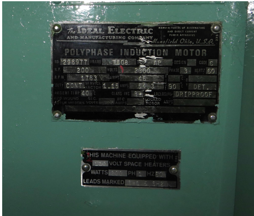
RESTON PUMP STATION'S MOTOR #1 NAMEPLATE
