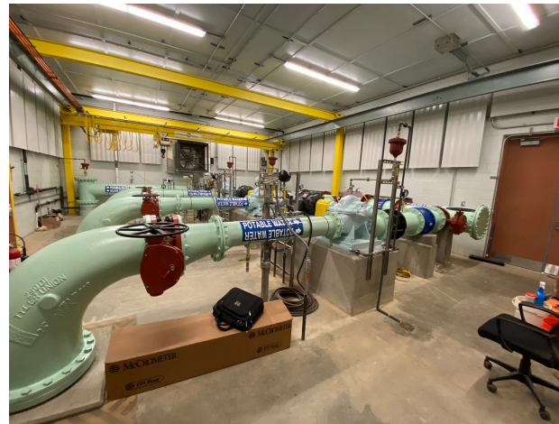
Inside view of the Sleepy Hollow Pump Station.
