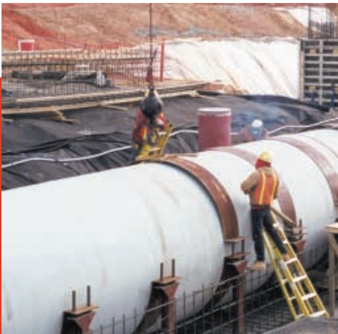
Workers at the construction site of the Griffith Water Treatment Plant install a 96-inch filter drain.
